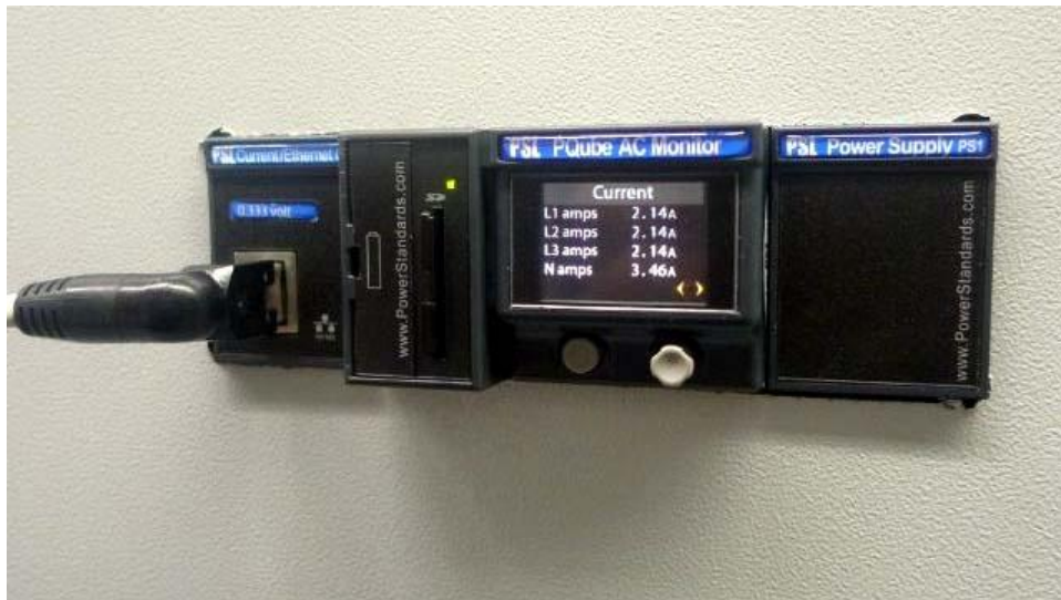
Photo 2 - Sample Caption - PQube installation at sample customer
