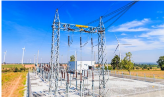
Substation partial discharge
